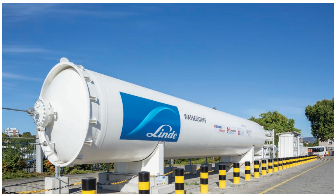
Figure 5.3 A pressurized hydrogen storage tank
