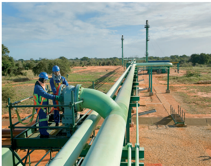
SASOL gas pipeline (Mozambique). Source: wikimedia
