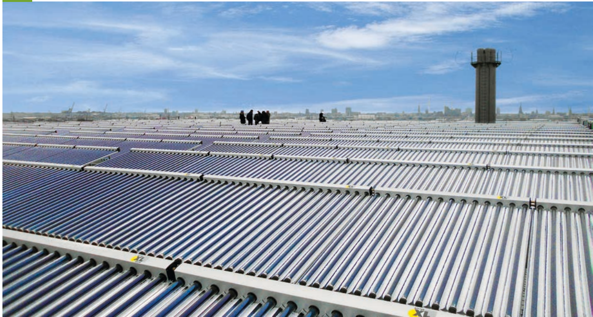
Energiebunker Wilhelmsburg, Hamburg, Germany Source: Ritter XL Solar, Photographer Oliver Killig
