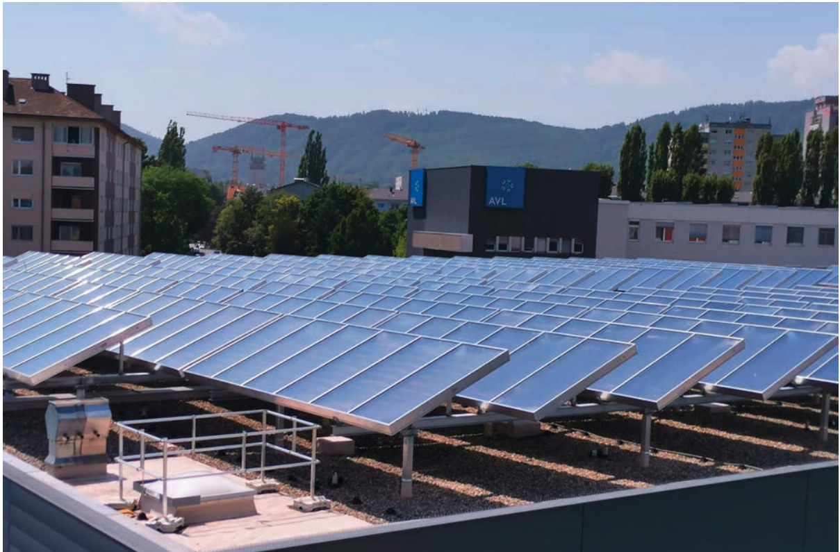
3,500 m 2 flat plate solar collectors supply heat to drive a 660 kW absorption chiller at the company AVL in Graz, Austria
