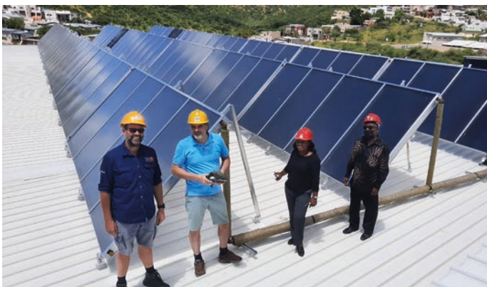
Partial view of the solar installation on Lady Pohamba Hospital in Windhoek, Namibia Photo: AEE INTEC
