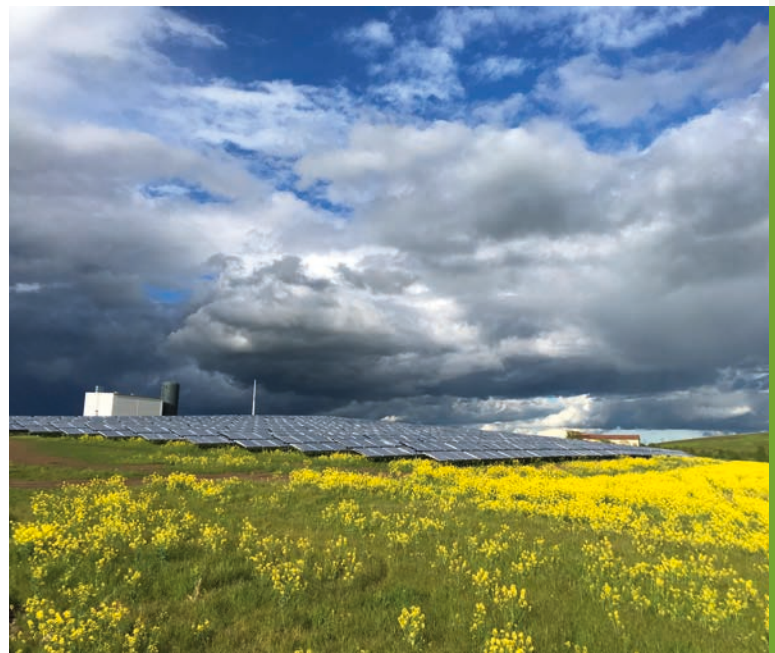
Municipal district heating network in Mühlhausen, Germany with 5.691 m 2 collector area
