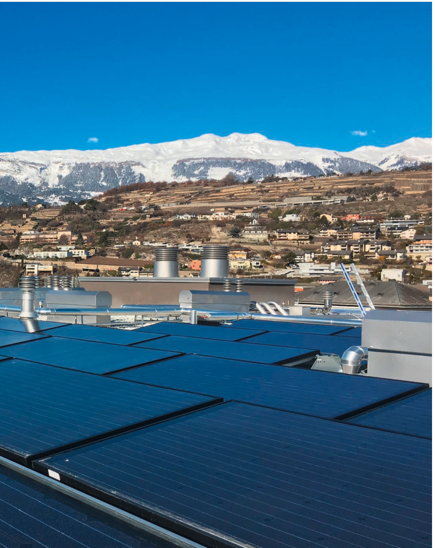
Sion, Switzerland. 41 PVT collectors on a building in the city center (sustainable building with Minergie label) Photo: DualSun, Switzerland
