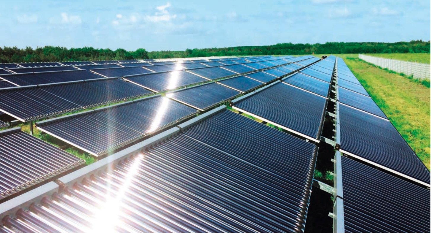
Solar District heating system with 18,732 m 2 evacuated tube collectors in Greifswald, Germany Photo: Ritter XL Solar
