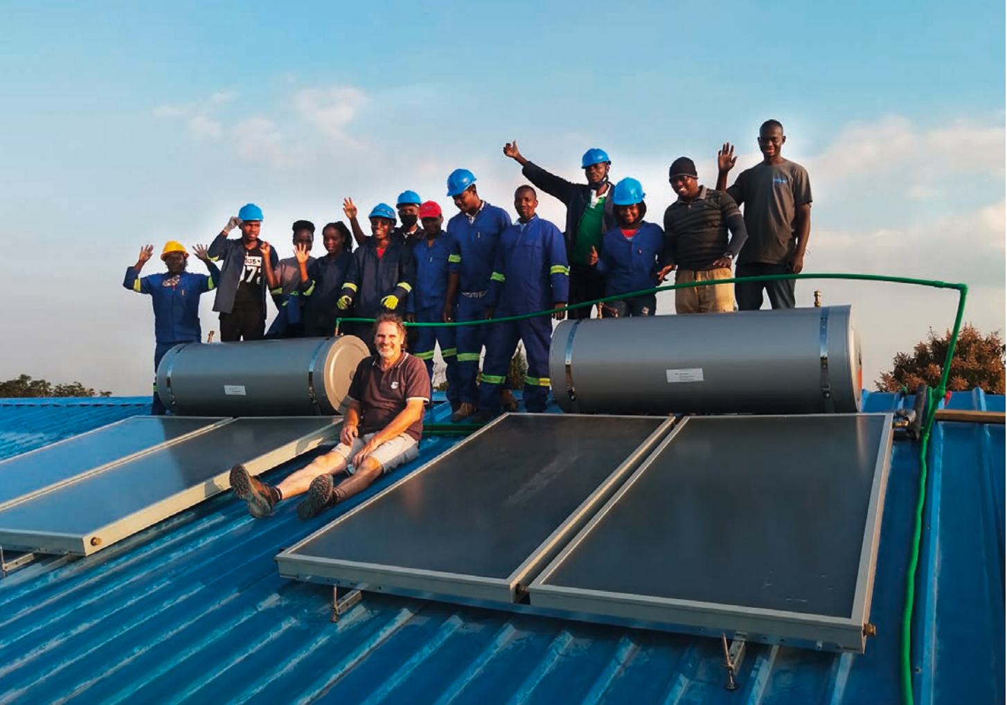
Thermosiphon systems in Mozambique Photo: AEE-INTEC
