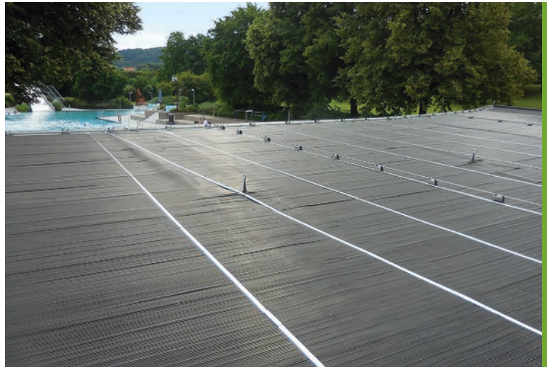
Solar system for outdoor pool Obersulm, Germany Photo: AST Eis- und Solartechnik GmbH, Austria
