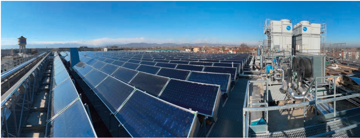
Solar process heat system for Martini & Rossi with a capacity of 0.42 MW th and equipped with high-vacuum flat plate collectors in Turin, Italy Photo: TVP Solar, Switzerland
