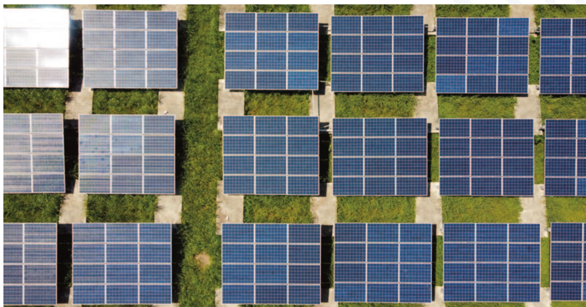
2 MW, Taipei Energy Hill, Taiwan.
