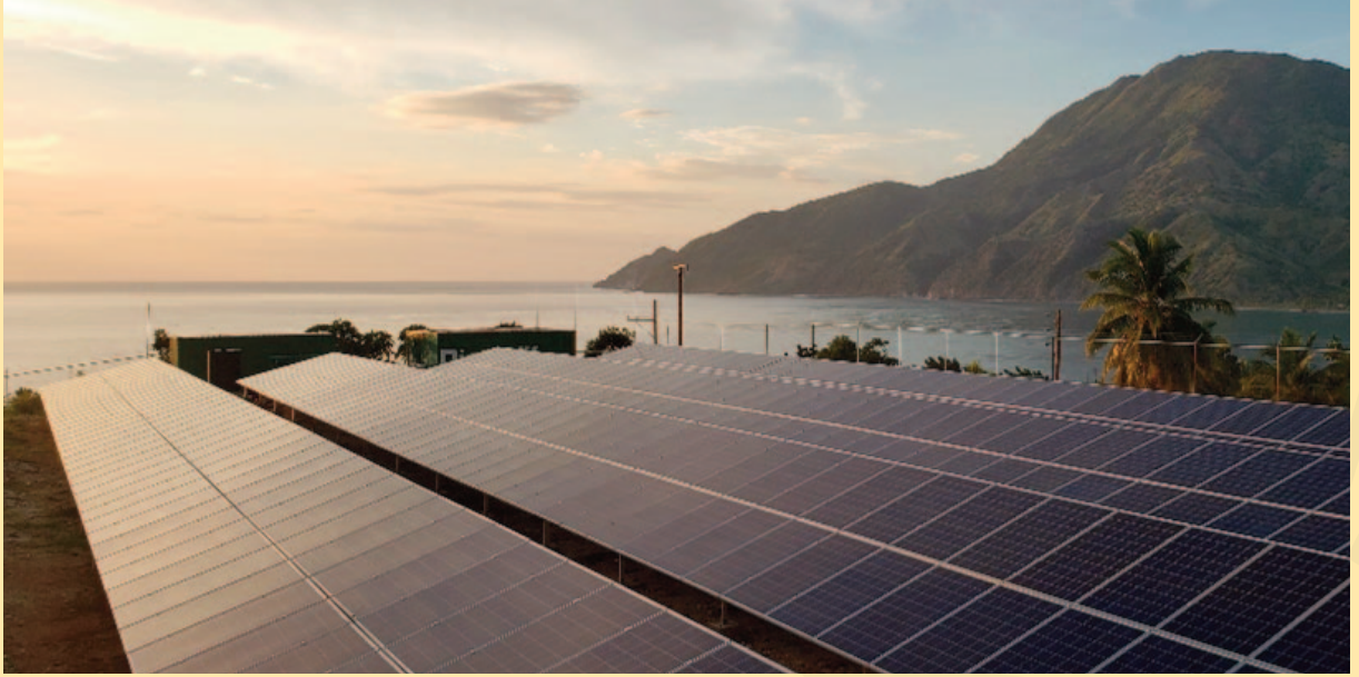
EarthSpark International's 95 kW solar array in Tiburon, Haiti basks in Caribbean sunshine.
