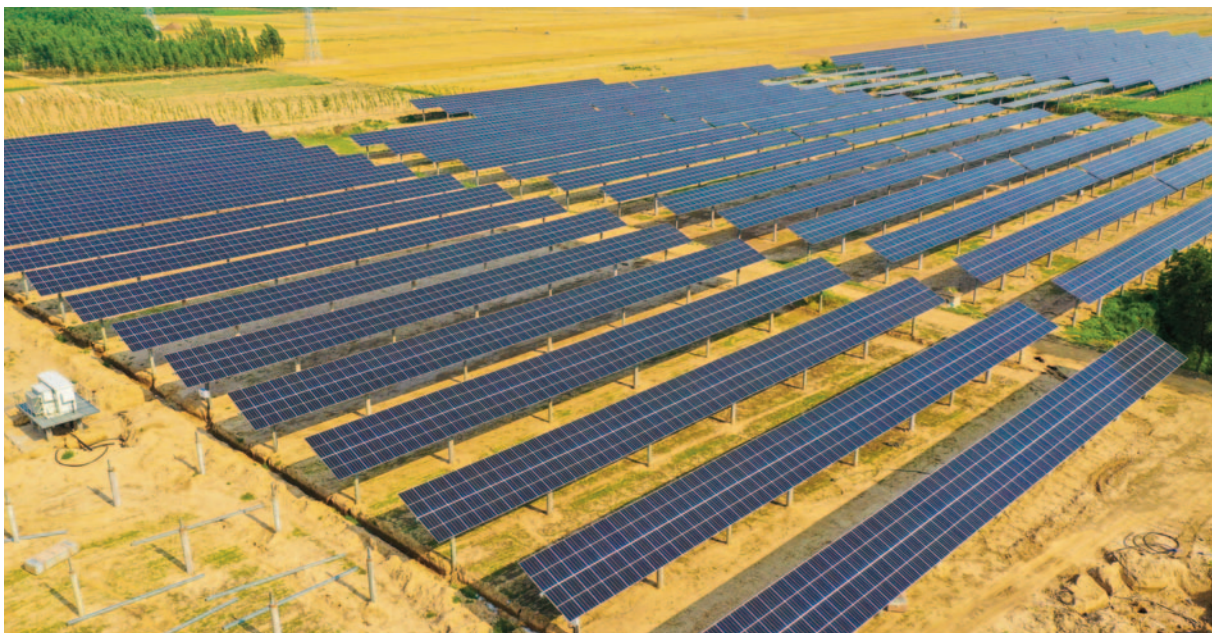
400 MW, Nangong, HeBei Province, China.
