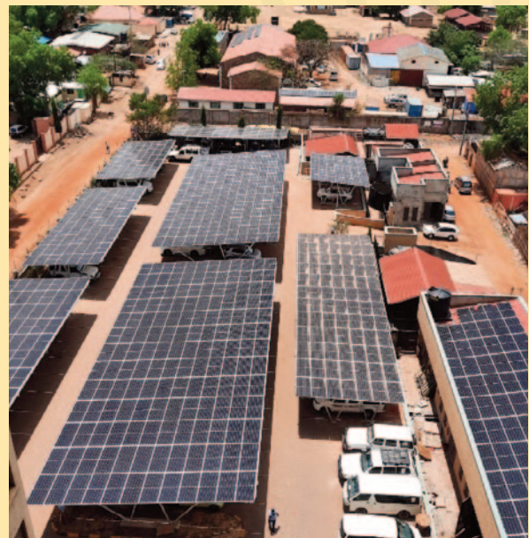
The new carport off-grid system for UAP Old Mutual Equatoria Towers, Juba, Sudan.
