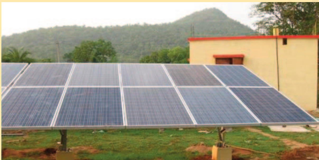
30 kW solar-powered Smart Nanogrid in Chhotkei, Angul, Odisha, India.
