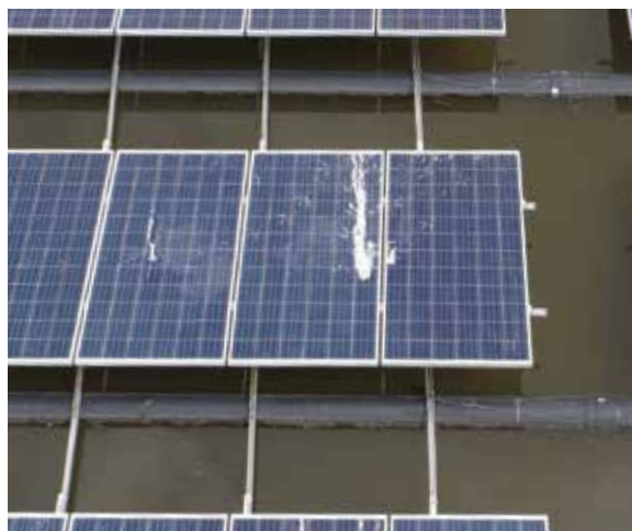
FIGURE 9.5 Severe bird droppings at a testbed in Tengeh Reservoir, Singapore
