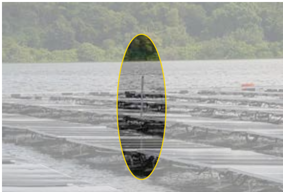
FIGURE 4.15 Air terminal rods installed on an FPV island, Singapore Tengah Reservoir testbed
