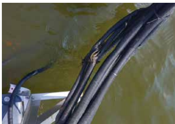
FIGURE 9.18 Conduit and cable sheath wear out
