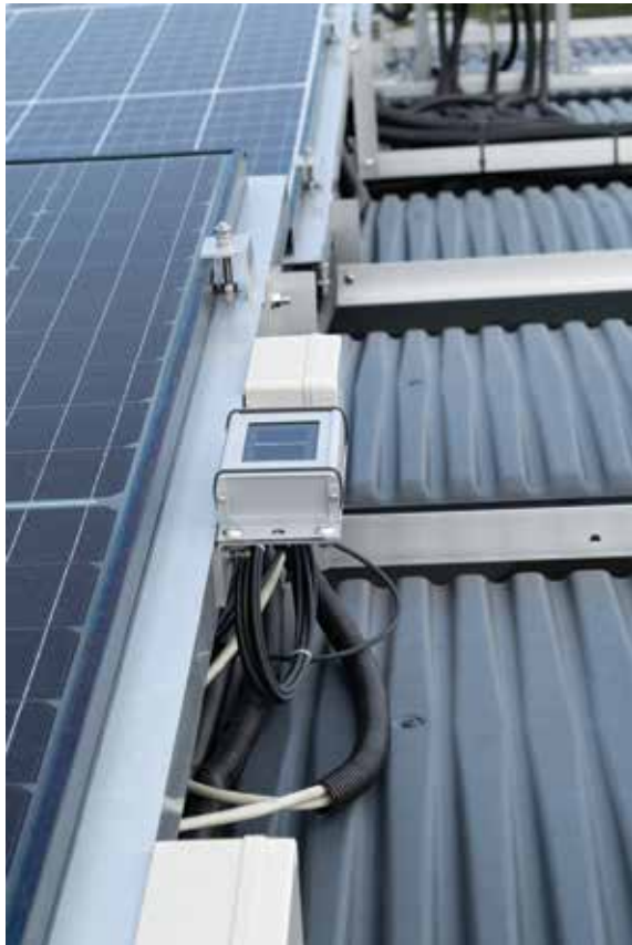
FIGURE 9.3 Irradiance sensor installed in the plane of the solar modules
