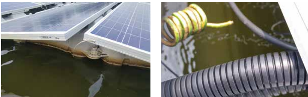
FIGURE 9.20 Bonding tapes/wires snapped due to constant motion of floats and excessive slackness
