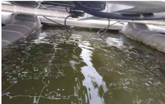
FIGURE 9.15 Connectors and cables submerged in water
