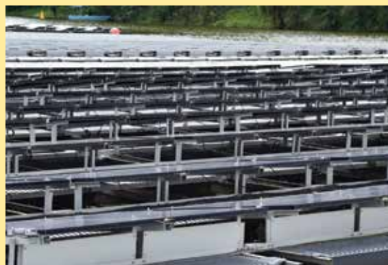
FIGURE 4.5 Windshields on the perimeter row of floats
