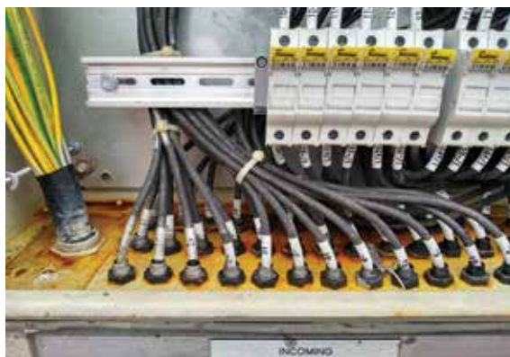
FIGURE 9.19 Water ingress and IP integrity compromised
