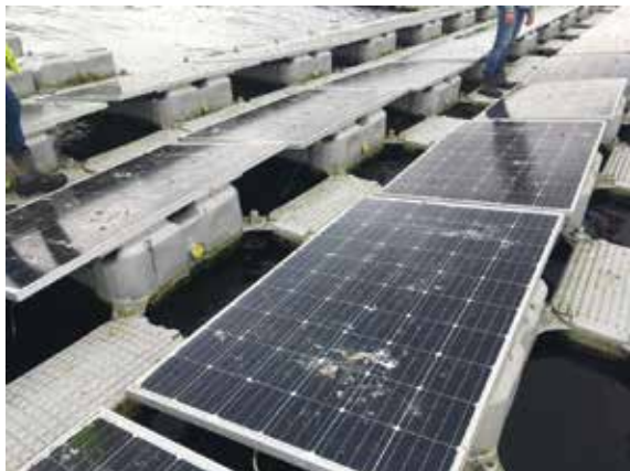
FIGURE 3.2 Severe bird droppings on an FPV project in the United Kingdom
