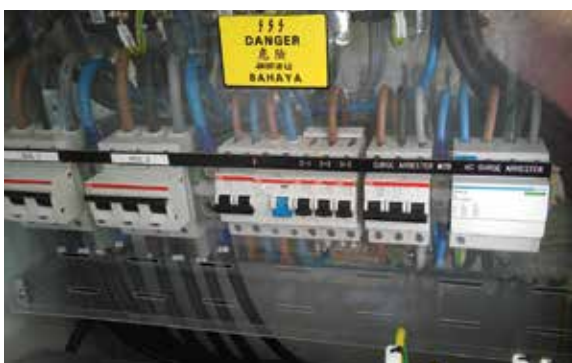
FIGURE 8.9 AC subboard with surge protection device
