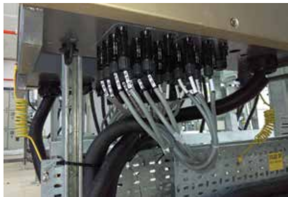
FIGURE 8.7 DC isolator switch at bottom of the inverter, and neatly terminated cables with labels
