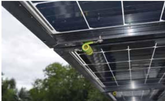
FIGURE 4.17 Equipotential bonding, Singapore Tengah Reservoir testbed
