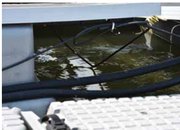
FIGURE 7.6 Examples of cables in contact with water
