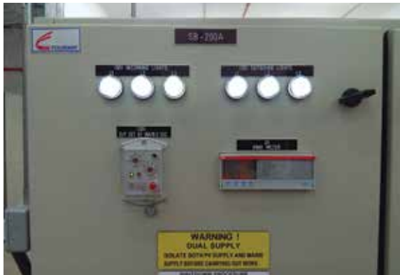
FIGURE 8.8 LED indicating grid supply and FPV supply
