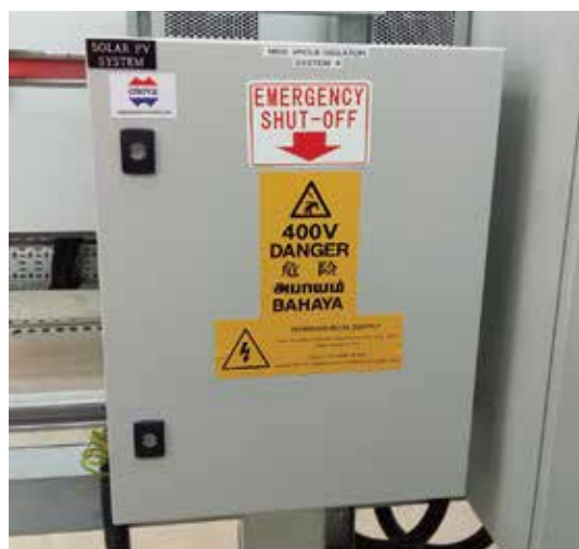
FIGURE 8.11 AC isolator with emergency shutoff
