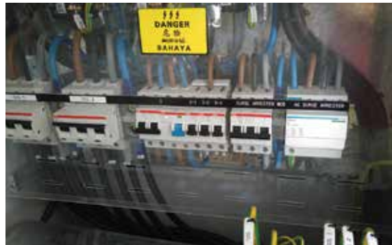
FIGURE 4.16 AC surge arresters installed on the AC electrical subsystem, Singapore Tengah Reservoir testbed
