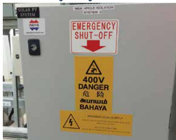
FIGURE 8.1 Safety warning labels
