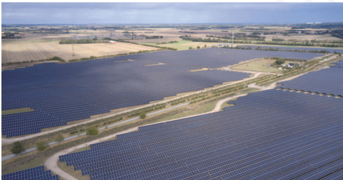
The 304 MWp Kassø PV plant was grid connected in 2022 to the 165 kV side of one of the main TSO transformer stations in the southern part of Denmark. It is constructed with half a million bifacial modules. In 2023 it will be connected to a 50 MW electrolyser and the world's largest e-methanol plant capable of producing 30,000 tons of green shipping fuels per year.
