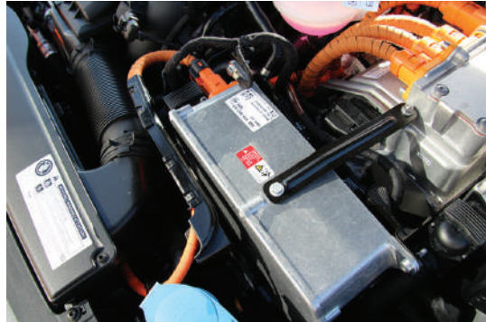
Figure 4.32 Orange cables and warning stickers on a Golf GTE
