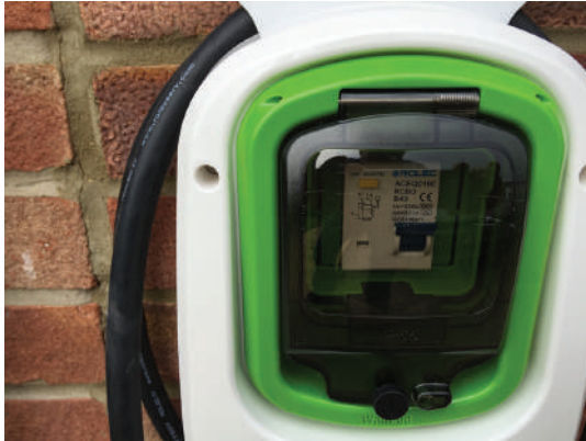
Figure 7.29 Domestic wall box mounted outside, with a permanent cable attached. It includes a residual current circuit breaker
