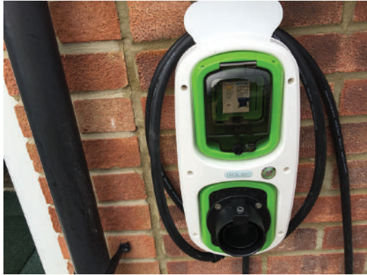
Figure 7.4 Domestic charging point
