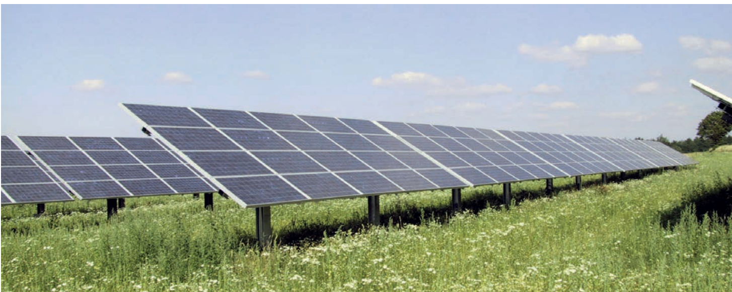
Fig. 7: Typical ground-mounted PV system. © Fraunhofer ISE
